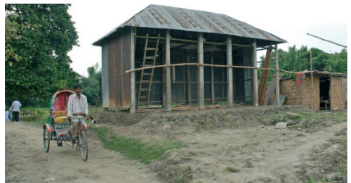
The basic structure of a typical Grameen house can be built expeditiously.
